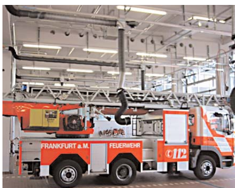
MAGNA TRACK® in Fire engine hall 1
